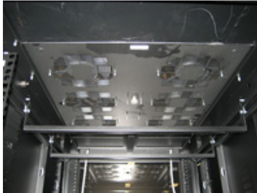
Figure 14: This shows the inside of the rack, looking up at the fan tray before modifications
