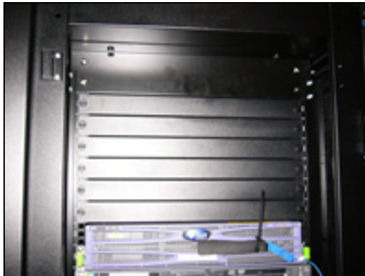
Figure 15: Essentially the same view as in Figure 14, but with the blanking panels in place. Also note the temperature sensors at the inlets of the highest server that were used during the validation testing
